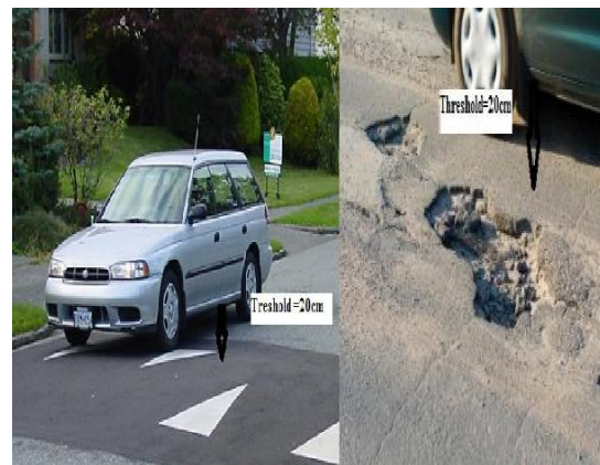
Fig. 6. (a) Detection of hump (b) Detection of pothole
