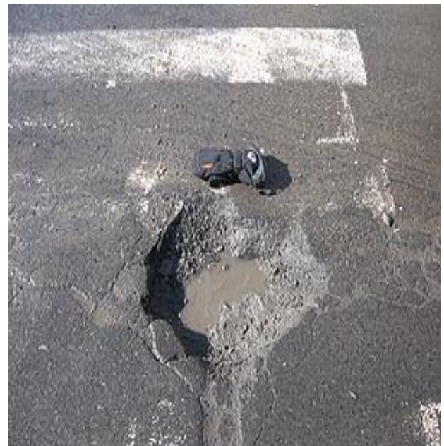
Fig.1. Pothole present in the road
